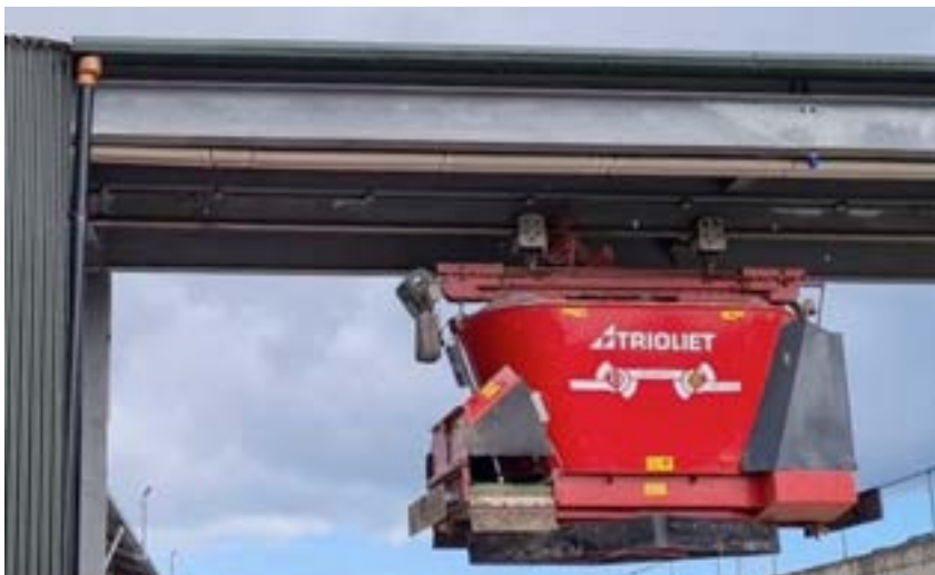
The overhead automated robotic feeding system mixes and delivers the feed at Ballywalter Farms in Co Wexford
