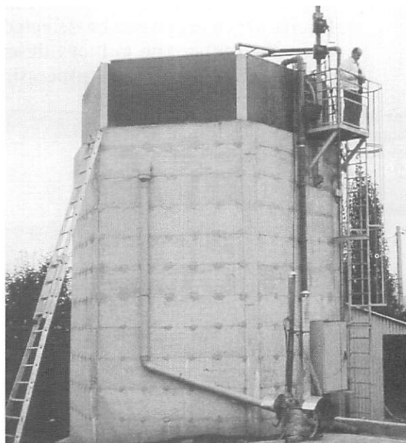
Fig 2. The aerobic/anoxic reactor.
