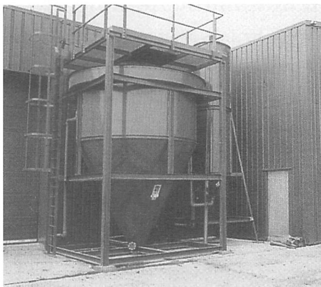
The clarifier for waste water treatment to meet NRA specifications.
