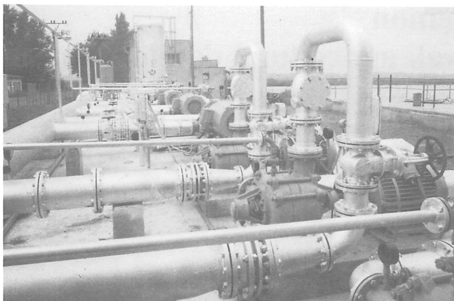
Open pumping station – Dyjávovice
