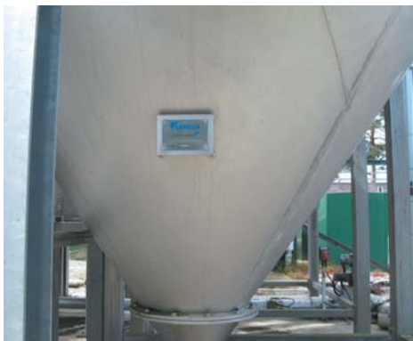
Cleaning out the wash-water Lamellas is a lot easier and less labour-intensive, due to the sludge hoppers at the bottom: it is very quick and easy to hose down the unit and drain out all the waste
