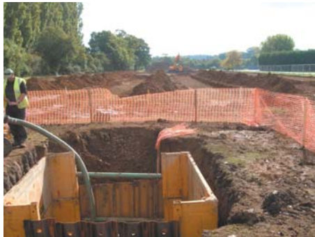
OCTOBER 2007 3.5m deep pumping chamber for lake de-watering and under liner drainage system
