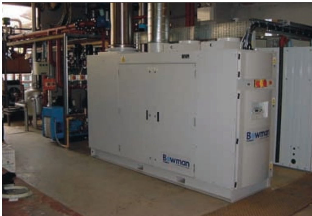
A trigenation system, where the heat is used to drive an absorption chiller to provide cooling
