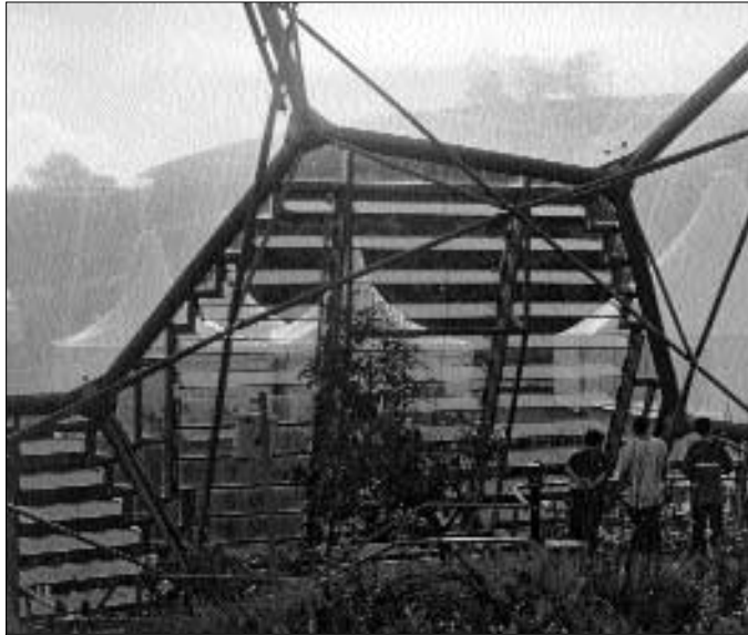
Looking out through one of the ground level louvred air ventilators, with one of the climate-control transducers (aspirated screen containing wet and dry bulb sensors) visible to the left of the small tree (Photo: John A C Weir)
