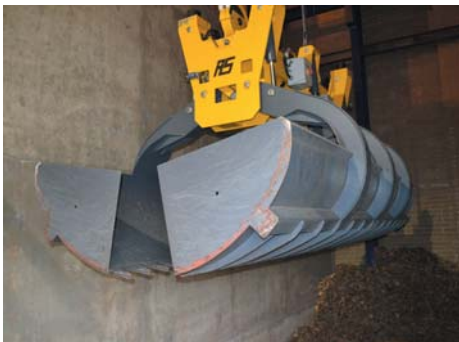
Figure 3. Automatic grab to feed chips to the drying section.
