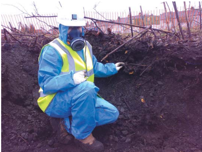
Ecologist supervising Japanese Knotweed excavation in asbestos impacted soils - the orange / yellow rhizomes are clearly visible
