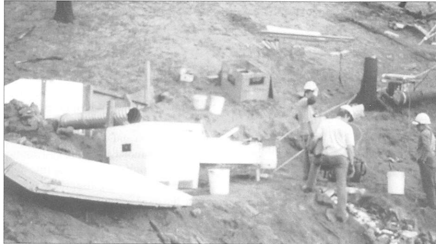
Fig. 9 Installing a weir and sediment collector on a site following a wildfire in the Wenatchee National Forest, Washington
