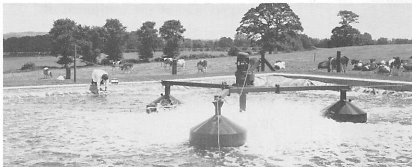
Reading University treatment plant for cow slurry: floating aerator.
